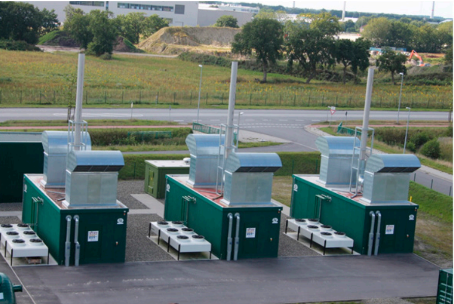
Figure A.55: CHP Generator
