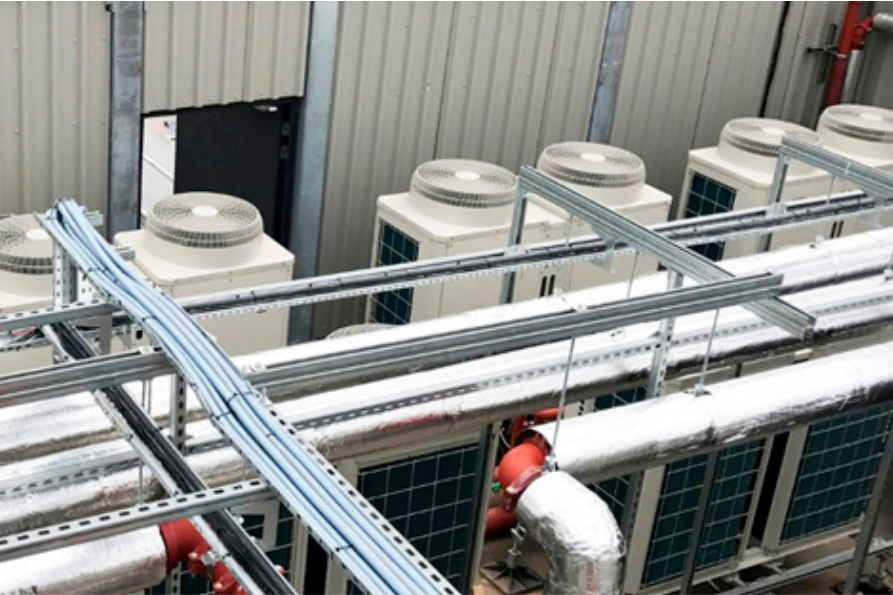
Figure A.56: Air Source Heat Pumps
